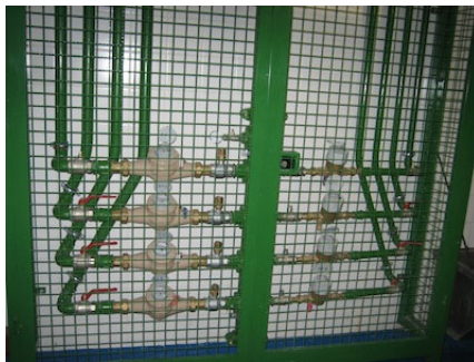
Water sectioning system used in a shopping center.
